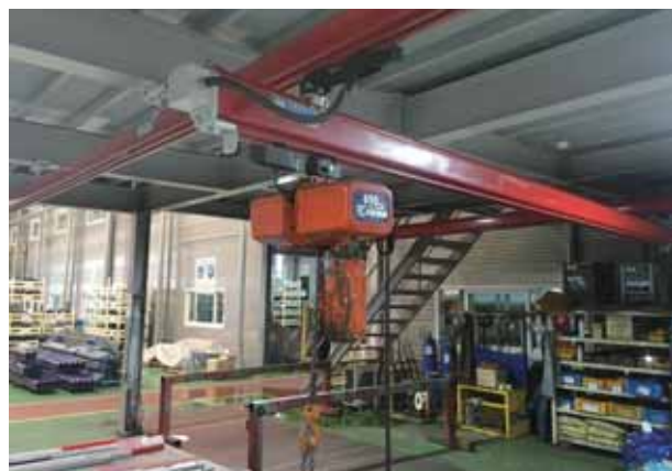
▲ Bus bar Track System
