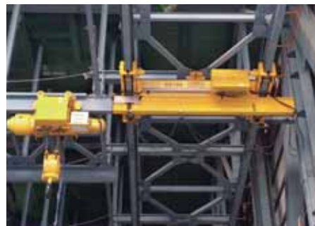
Pulverizer Maintenance Crane (Suspension type 40Ton)
