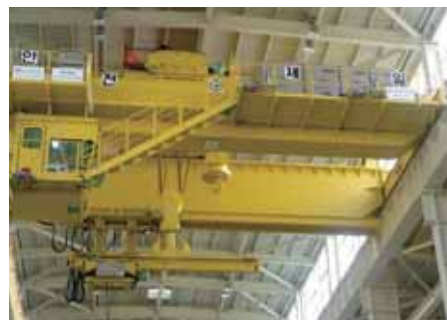
Steam Turbine Over Head Crane(120Ton)
