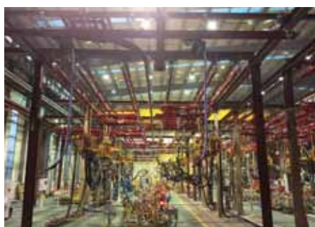
Bus Bar Track System (Car welding line)
