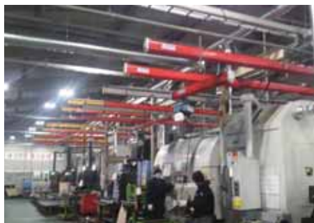
KH-Track system (Machining shop)
