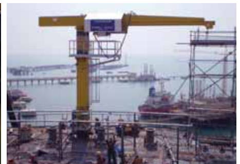
LNG/LPG Pump Lifter
