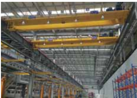
Over Head Crane
