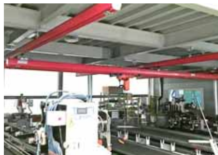
Bus Bar Track System (Welding shop)
