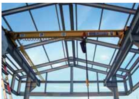
Air type Over Head Crane
